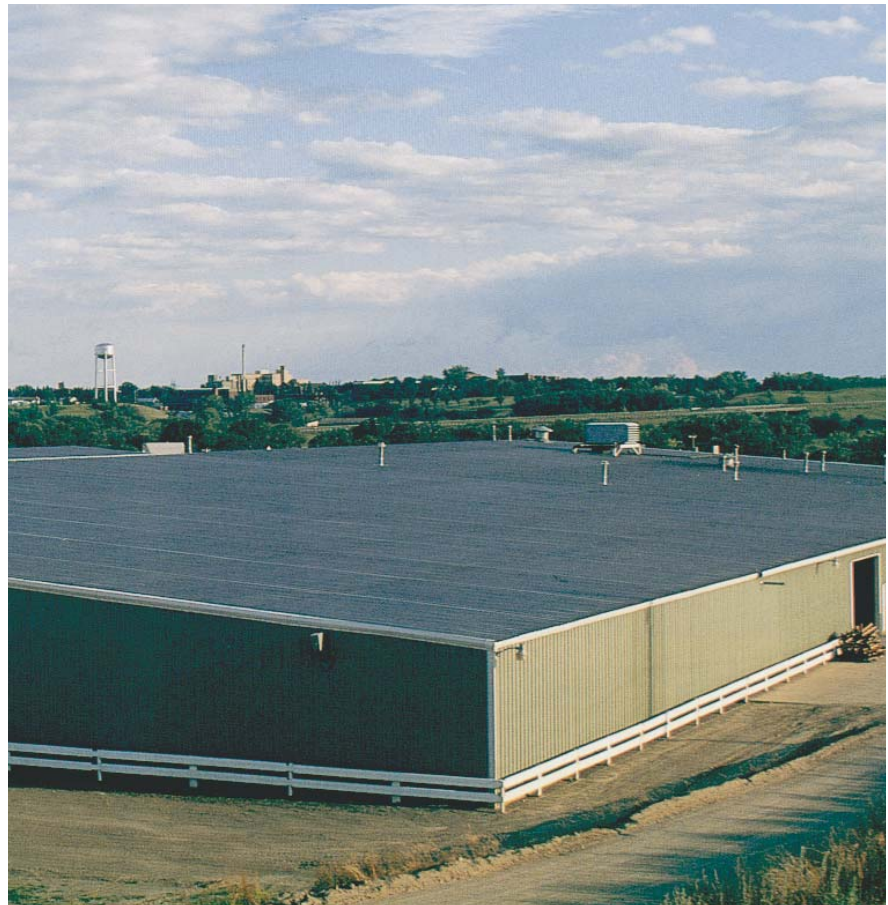
Starting in October, low-slope, unpainted roofs for temperature-regulated buildings will not qualify as a cool roof under the 2005 California Title 24 Energy Code because they do not meet reflectivity and emissivity requirements. To use metal roofing, either the envelope trade-off compliance method or the whole building performance compliance method must be used. The Cool Metal Roofing Coalition is lobbying for more input with the California Energy Commission, as it works on the 2008 Code. WEDGCR PHOTO
