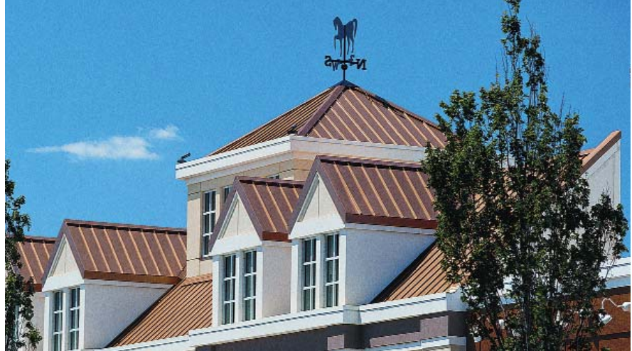
Copper Penny is one of the cool colors offered on Petersen Aluminum panels. The coatings on these snap-lock standing seam panels help make Bowie Towne Center a more energy efficient building. PETERSEN ALUMINUM PHOTO
